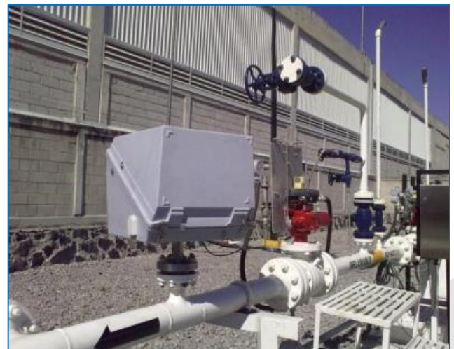
Figure 6 – Gas PTi pipeline mounted installation
