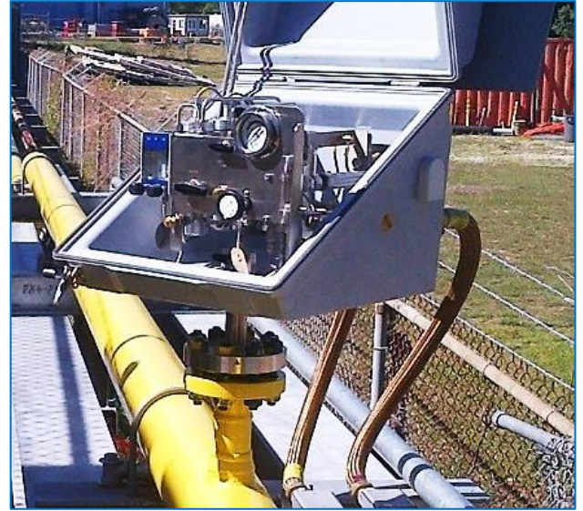
Figure 4 – Gas PTi pipeline mounted installation.
