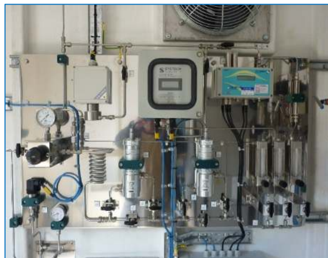
Figure 4 – Gas PT sensors installed in Biomethane kiosk
