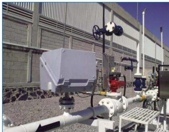
Figure 6 – Gas PTi pipeline mounted installation
