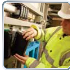
Remove defective unit and return for disposal
